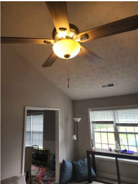
CEILING FANS Satisfactory Notes:
