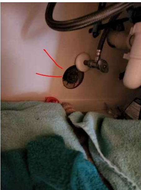
PRESSURE AT FAUCETS Satisfactory
